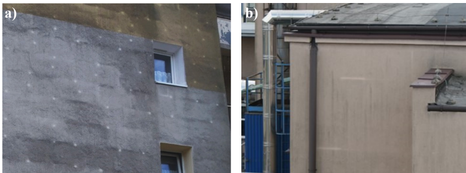
Fig. 4. Permanently soiled facades with acrylic plaster. Unsoiled surfaces in the area of: a) mounting pins, b) gaps between the panes ( own photos )
